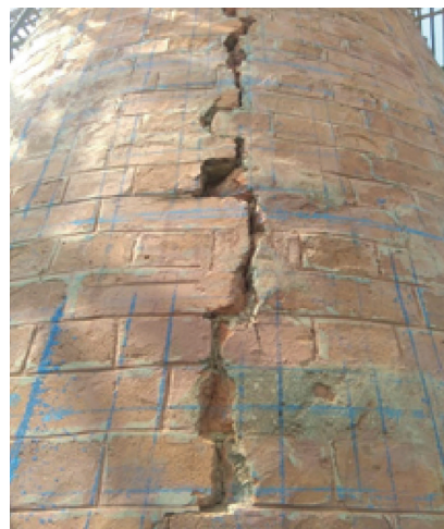
Figure 3: Assessment of crack on the stack.
