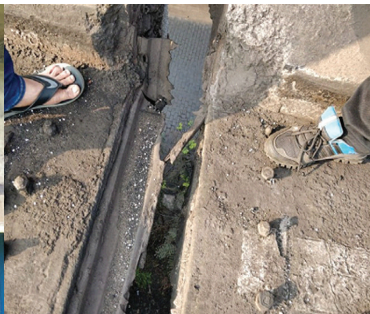
Fig.3: Condition Of Expansion Joint
