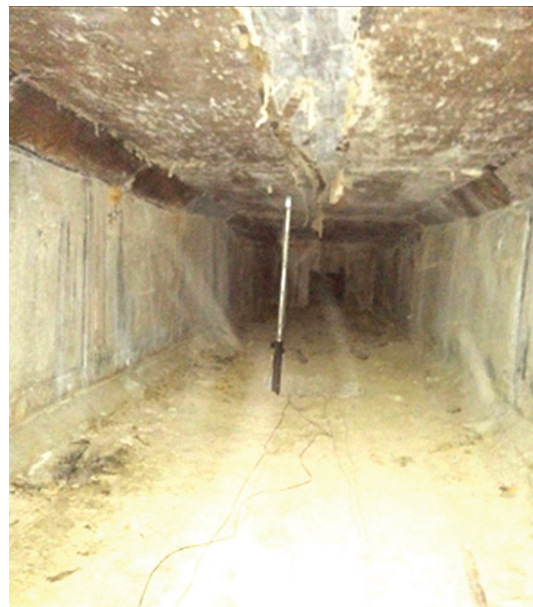
Fig. 16 : Sensor Inside the Box Girder
