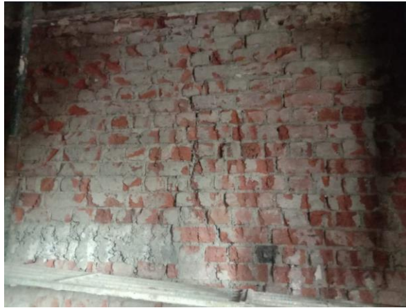
Fig 7: Image showing cracks in periphery brick wall
