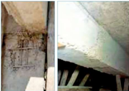
Fig. 4: Rebar Exposure and Honeycombing in Concrete
