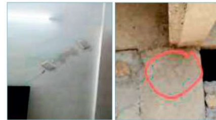
Fig. 3: Cracks in Structural Members
