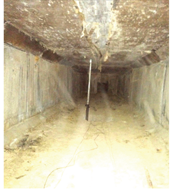
Fig. 16 : Sensor Inside the Box Girder
