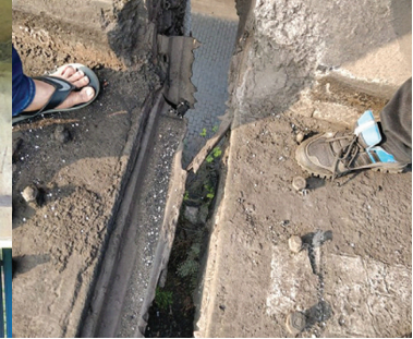
Fig.3: Condition Of Expansion Joint
