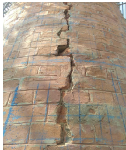
Figure 3: Assessment of crack on the stack.
