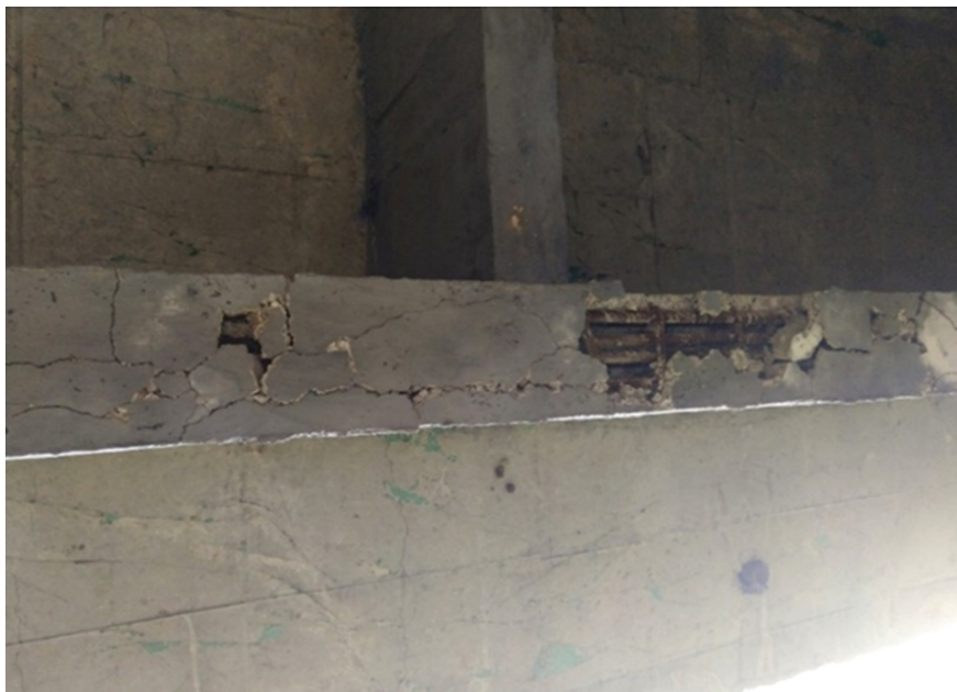
Fig.2 : Severely deteriorated girder, wide cracks, loose concrete, exposed reinforcement
