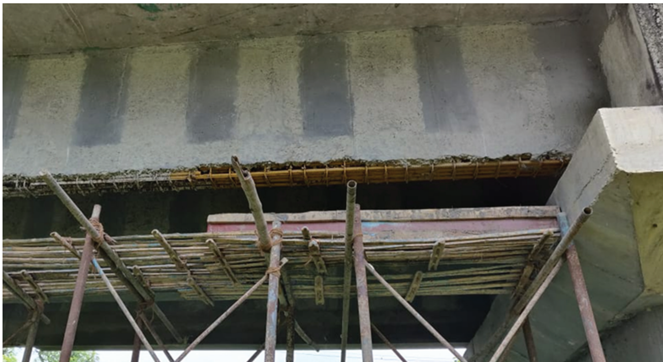
Fig. 10: Exposed Reinforcement and Anti-corrosive paint
