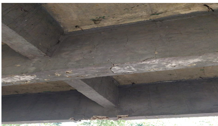
Fig 4: Efflorescent effect on Concrete and cracks in interior girder
