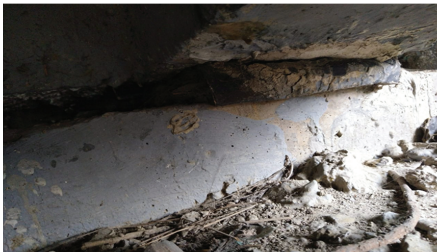
Fig 3: Severe deterioration in Concrete
