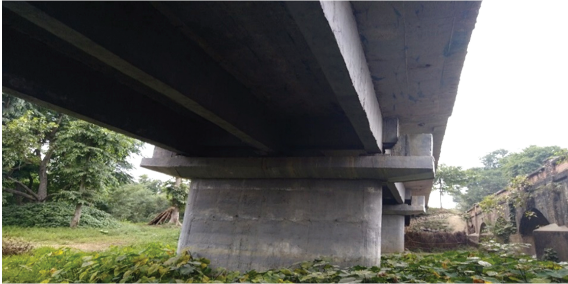
Fig 1: A view of damaged bridge.
