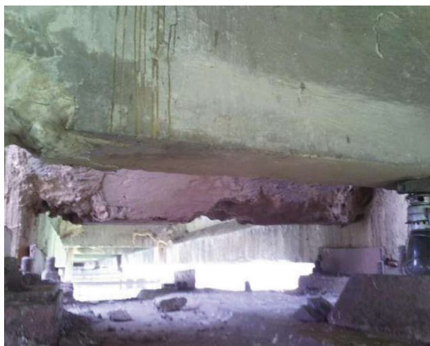
Fig. 5 Cracks and delamination at locations of bearings
