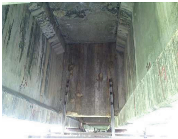
Fig. 4 Surface de-coloration and deterioration
