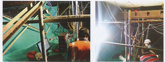
Fig 5: Wiring of Sensors near Data Acquisition Arrangement in Congested Site Area
