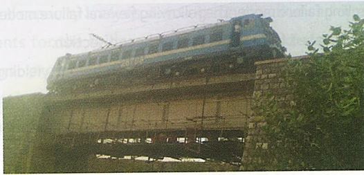
(a) Before Strengthening
