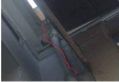
Fig 9: Major crack developed on the 1st floor as seen from outside
