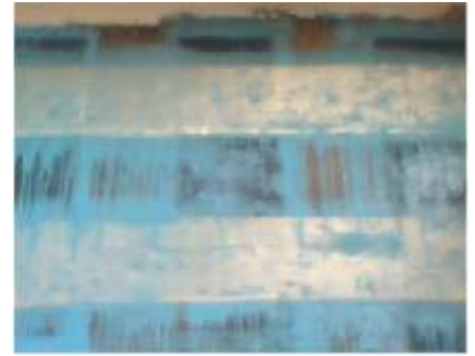
Fig 8: a) Vertical Application of C- FRP wrap and horizontal application of G-FRP.
