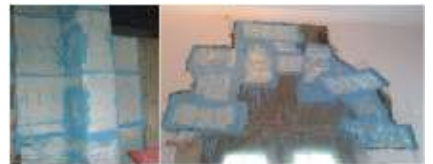
Fig 14: (a) Column Wrapping done for confinement and strengthening (b) Wraps done over the cracks for arresting them.
