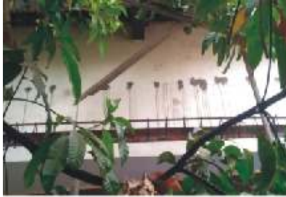
Fig 6: Horizontal Crack on the Structure.
