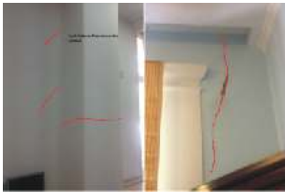
Fig 10: Cracks present as seen inside on the columns and on the top.
