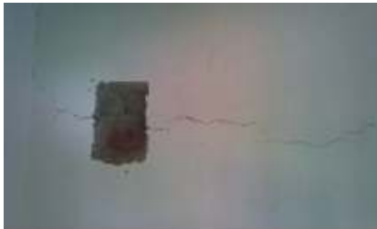
Fig 7: Horizontal Crack in the wall
