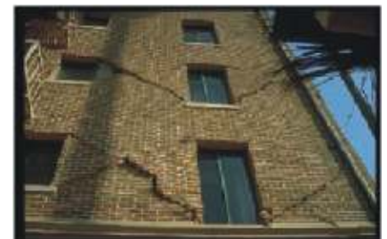
Santa Monica, Northridge Earthquake, 1994 Fig 3: Cracks developed in the earthquake.
